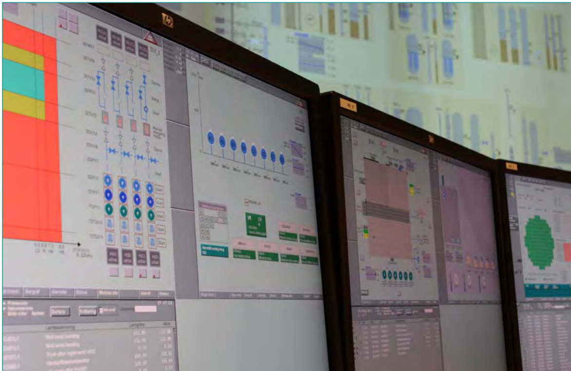
Various HSI prototypes installed and tested in HAMMLAB.
