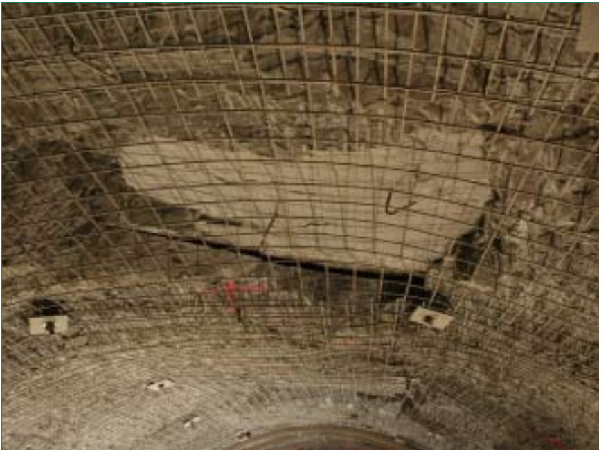
Fig. 5: Platy slab in the ceiling which developed with distance to face and collapsed later on.
